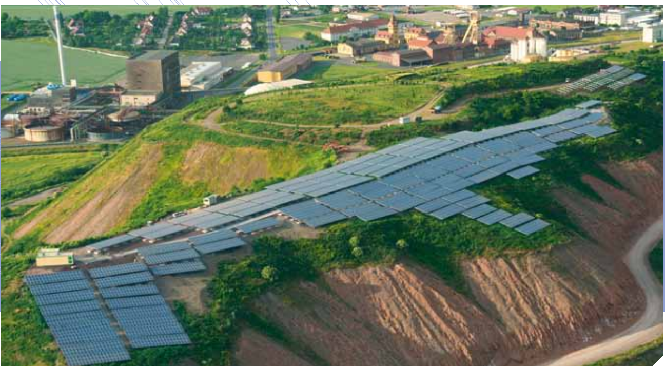
Example of a special construction: Ground level arrangement with concrete foundations and rotary foundations (under construction) on a potash waste dump as a rain protection for the prevention of the ground salinisation
